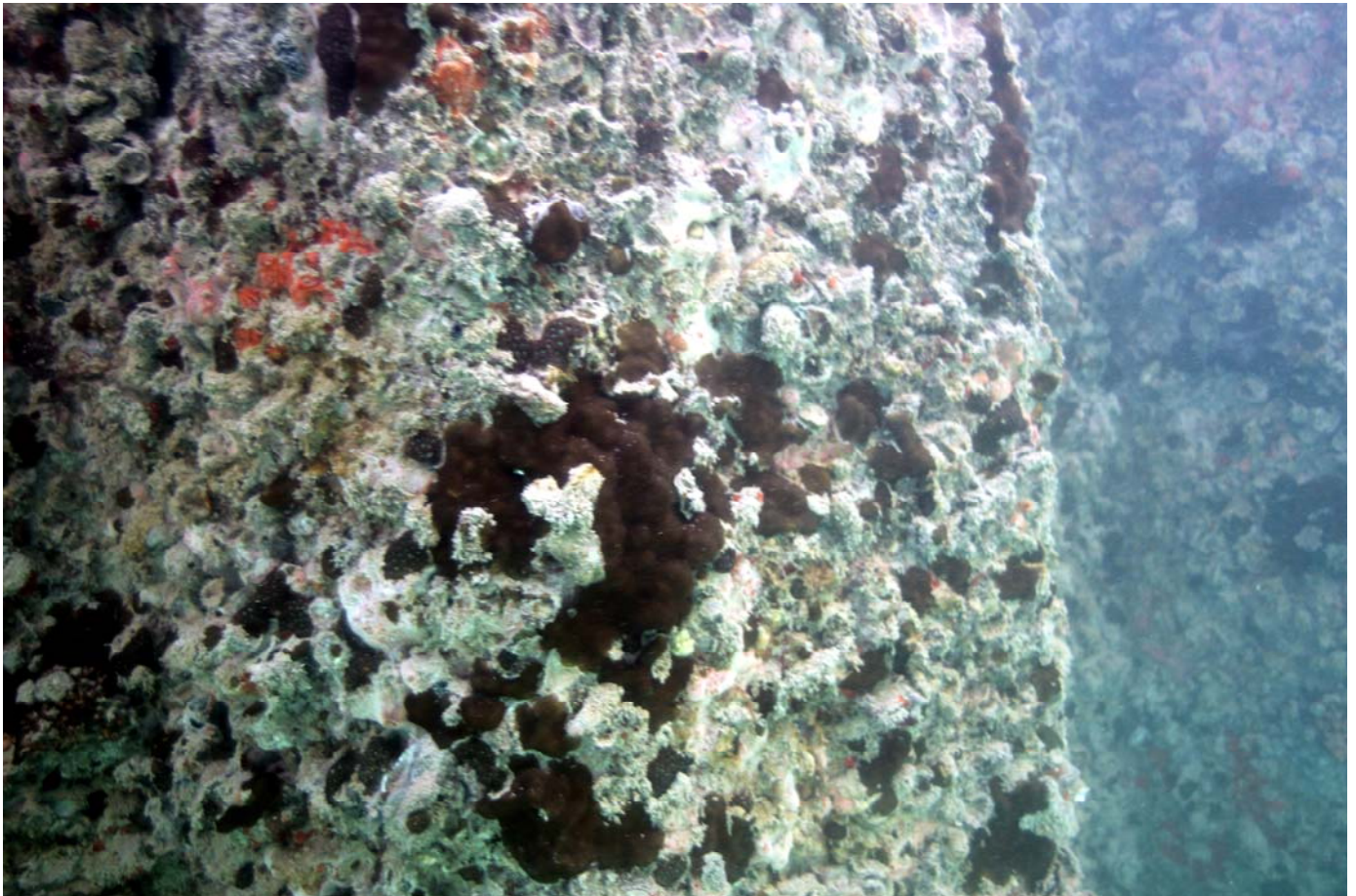
FIGURE 4. Two photos of sheet-piling wall of Pier 41 designated as Section H-3 in Figure 1 under moored commercial boats. Predominant corals in this section were small encrusting colonies of Porites lobata in both top and bottom photos.
