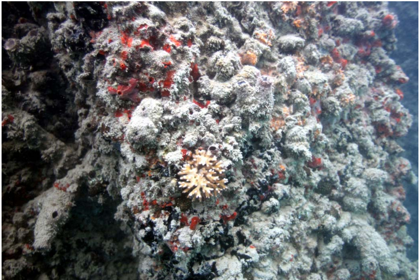
FIGURE 2. Two photos of sheet-piling wall of Pier 42 designated as Section H-1 in Figure 1 inshore of PSI dry-dock KeKaulana. Predominant corals in this section were small branching colonies of Pocillopora damicornis as seen in bottom photo.
