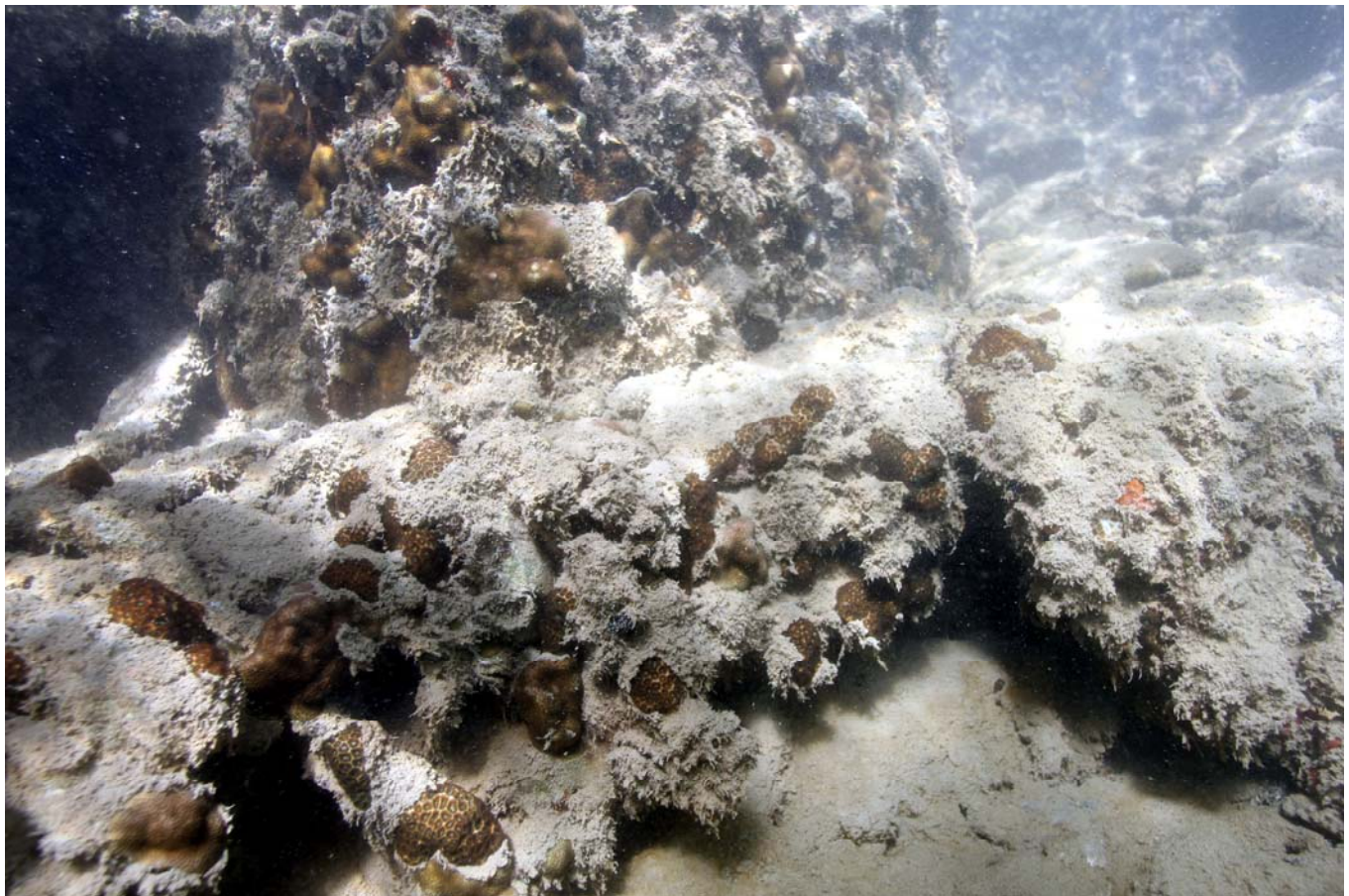
FIGURE 3. Two photos of sheet-piling wall of Pier 42 designated as Section H-2 in Figure 1 under moored commercial boats. Predominant corals in this section were small encrusting colonies of Porites lobata (top photo) and Leptastrea purpurea (bottom photo).
