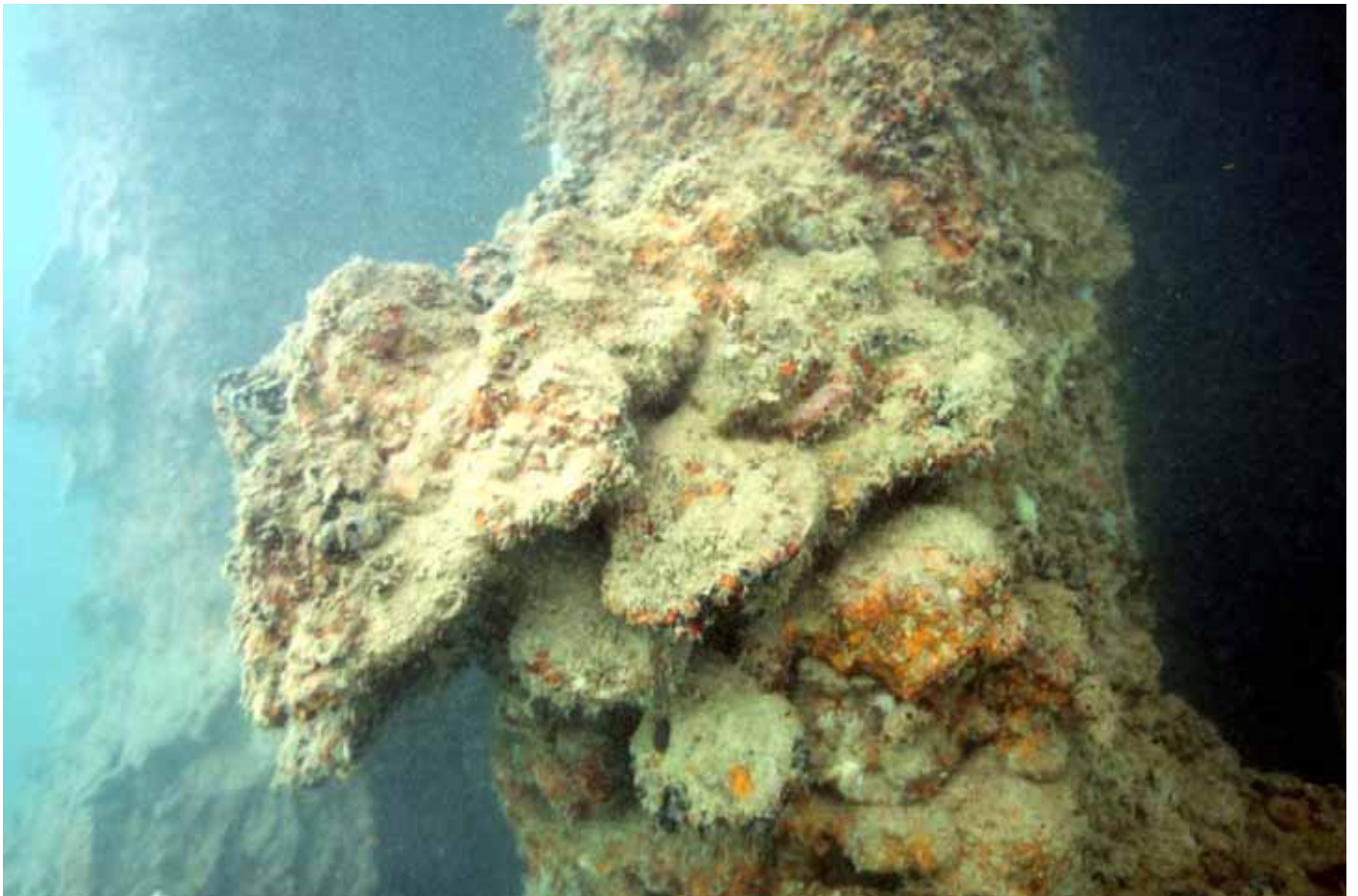
FIGURE 42. SECTOR P-26. Colonies of predominantly dead Montipora spp. on pilings comprising Pier 26. Small colony of M. capitata in top photo may be either the resulting remnants of partial mortality of a large colony or settlement of growth of multiple new colonies on older remnant structure. For location of Sector P-26, see Figure 6.
